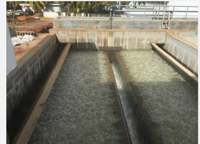
Testing - washing cycle running
