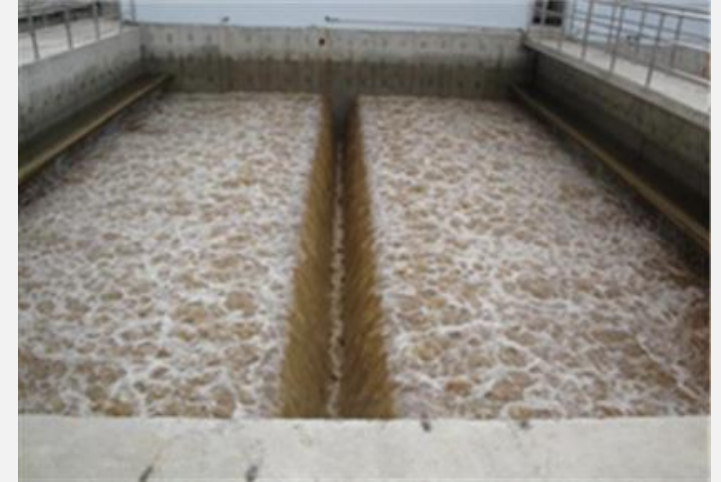
Filter in Backwash Mode
